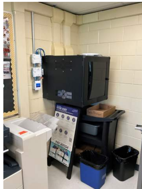
01 CLASSROOM BUILDING 'D' - IDF
