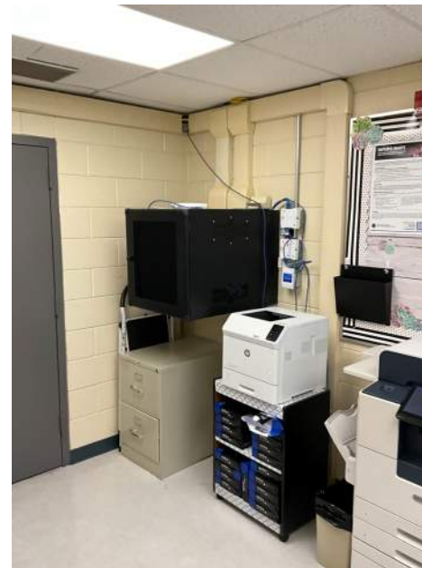
01 CLASSROOM BUILDING 'E' - IDF
